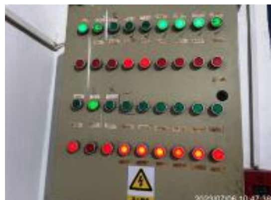
Distribution box with warning sign.JPG
