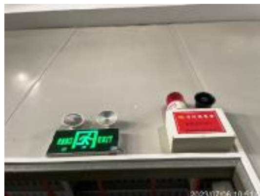
Exit sign, emergency light and fire alarm.JPG
