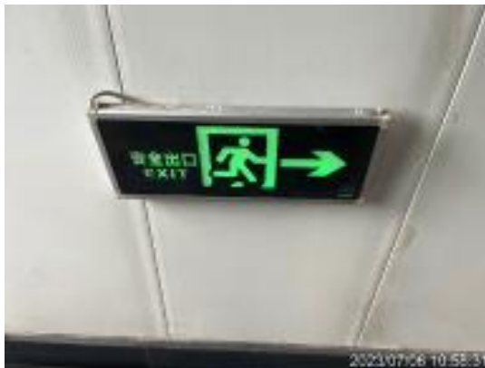
Evacuation indication sign.JPG
